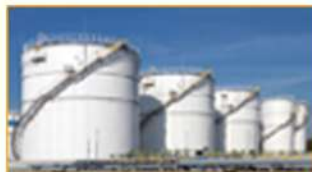
Oil/Gas Storage Tanks
